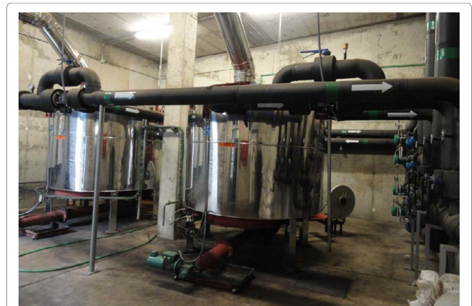
Figure 2: Thermal power plant installed at a Public Health administration building in Mérida (Badajoz).
